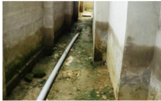
Figure 5b. Green stain on external wall
