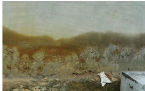
Figure 5d. Brownish-yellow stain on external wall
