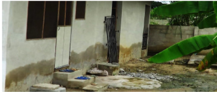
Figure 7a. Walls in the southern orientation showing signs of dampness
