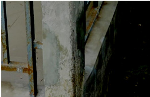
Figure 5a. Crack in column
