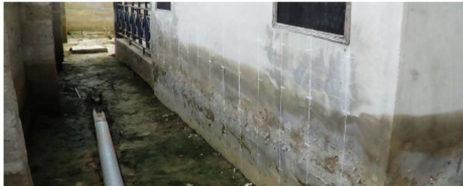
Figure 8a. Eastern orientation showing signs of dampness
