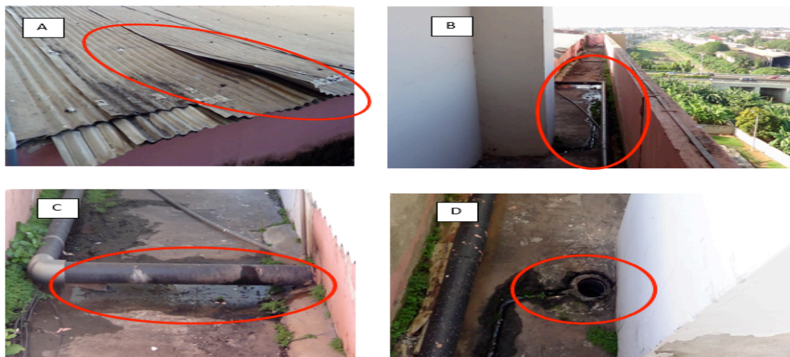
Figure 8: Slipped roofing sheets (A), leaking drainage pipes (B and C), Discontinuous discharge pipe (D)
