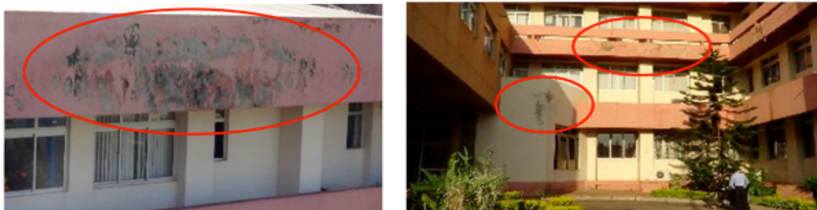
Figure 2a: Peeling of paint resulting from the direct exposure of the building to sunlight, wind and rain
