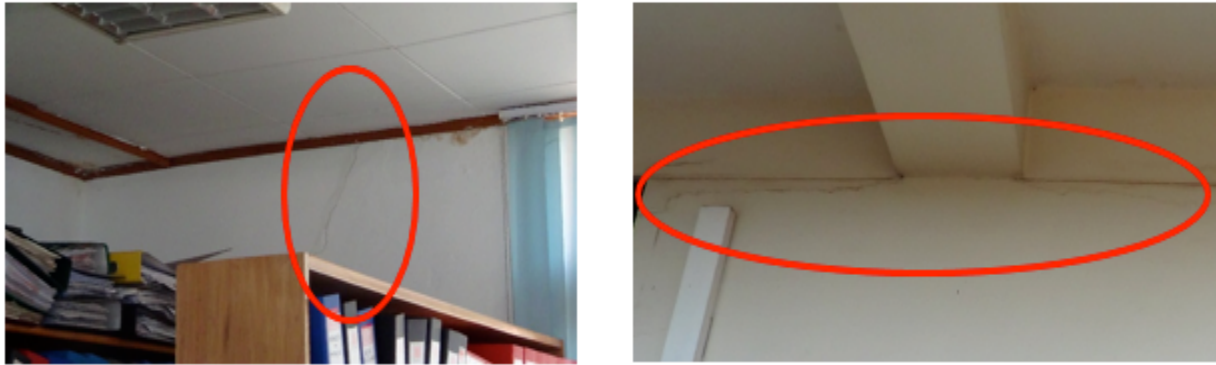
Figure 7: Diagonal (left) and horizontal (right) cracks on the interior walls of the building
