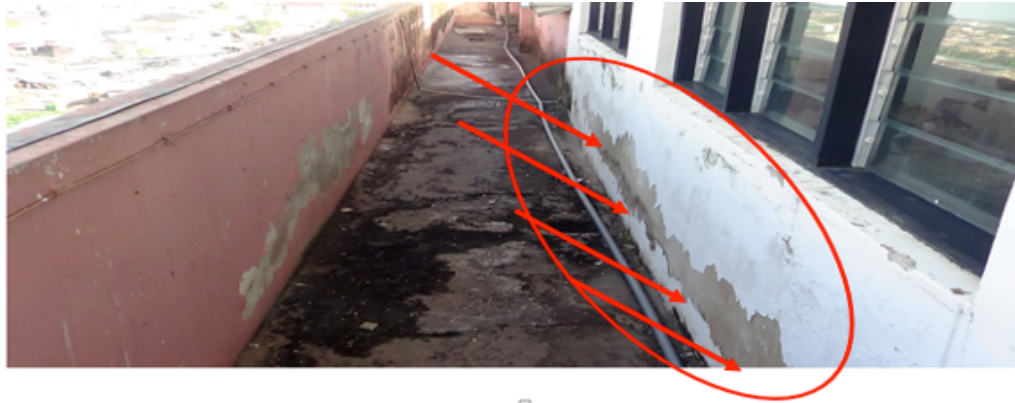
Figure 2b: Peeling of paint resulting from the action of moisture in the walls of the building
