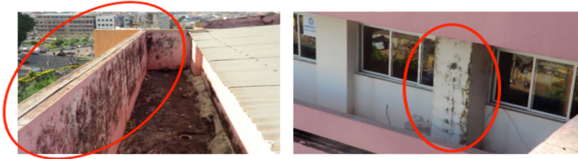
Figure 4 Stains and discolouring of walls
