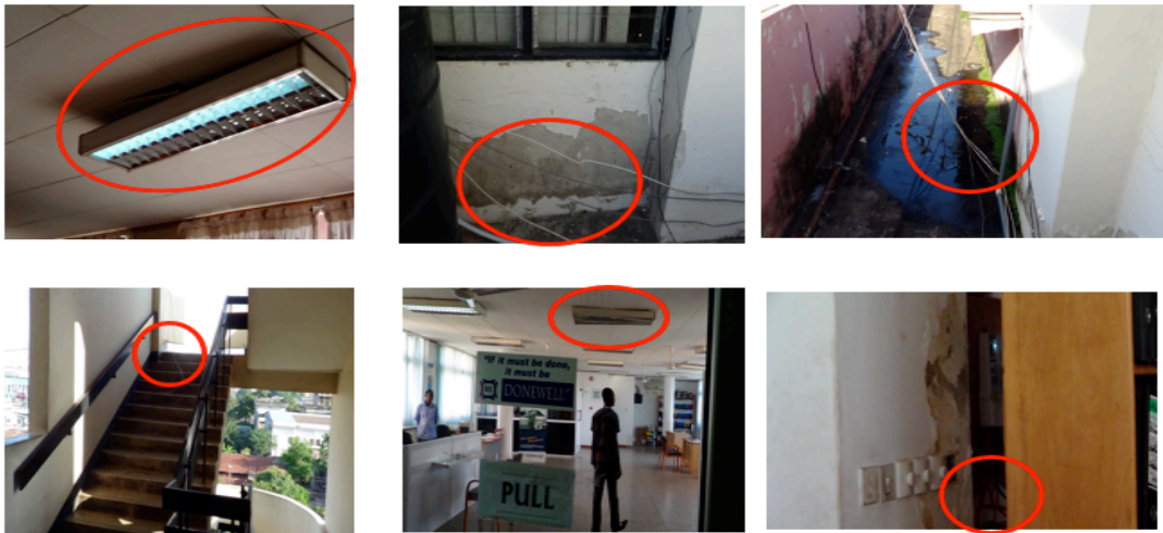
Figure 6: Faulty electrical fittings
