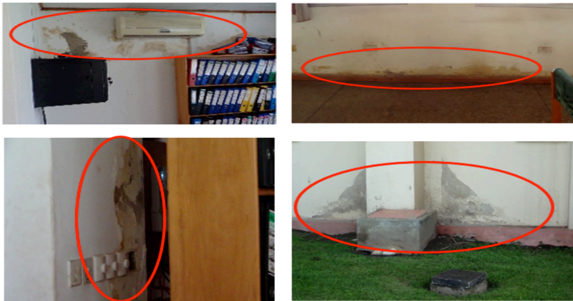
Figure 5a: Dampness resulting from water leakages and below ground water sources
