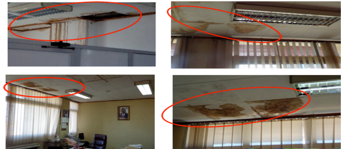
Figure 3a: Signs of ceiling leakages inside the building
