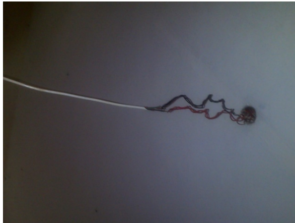
Figure 11: A room with illegal
