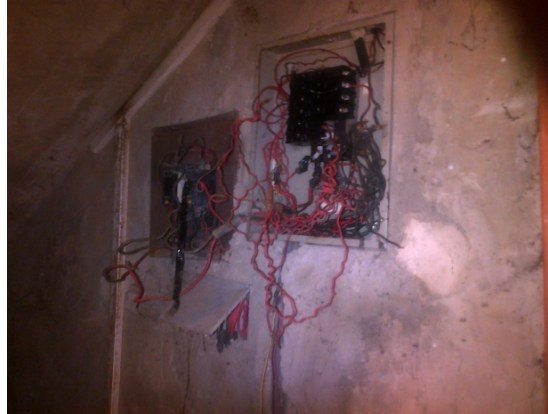
Figure 13: An exposed distribution board in the hostel
