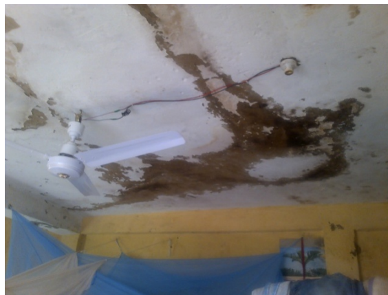
Figure 12: Room with illegal connection to fan electrical connections to socket
