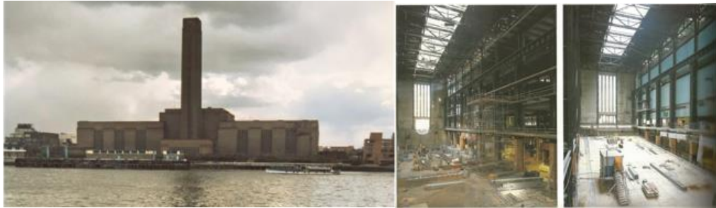
Figure 1: During the construction of the ramp in turbine hall of the old powerhouse station
